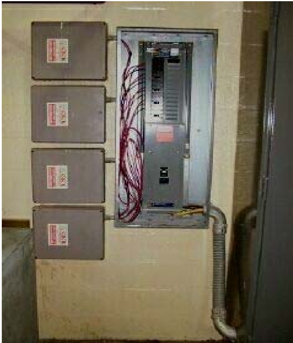
Figure 4. Bank of 4 USES Units connected to the H-10 Motor Control Center for 500 HP Compressor H-10 at Icelandic USA, Inc. Individual units are wired to individual 30 amp breakers and the connection passes through a 150 amp master breaker to the incoming power lugs in the MCC via the cable at lower right.
